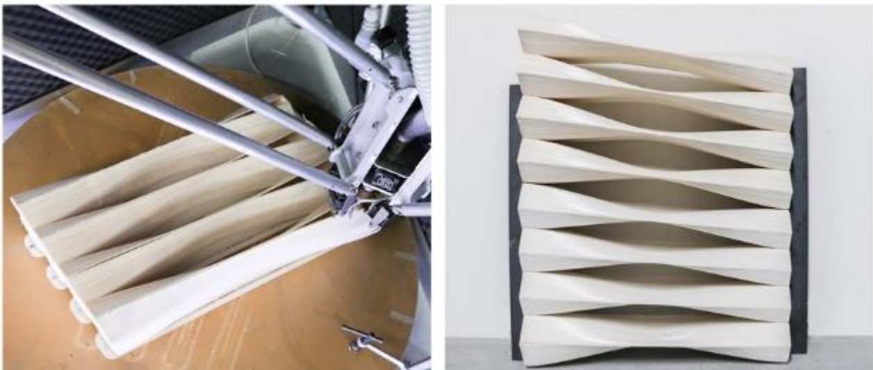
Figure 3: on the left the 3MT while printing the panel, on the right two panels assembled
